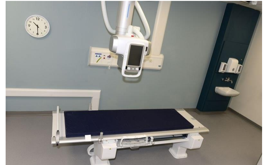
Above: A newly handed over NHS X-Ray room
